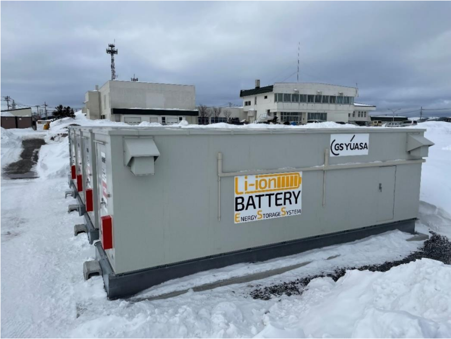
The power storage system in situ
