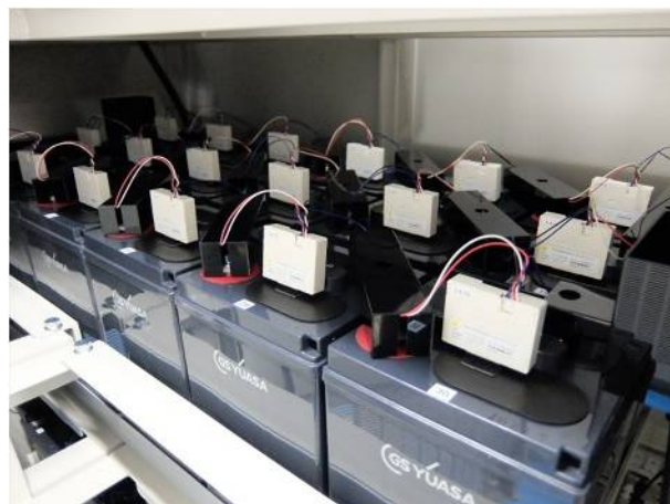
Example of installation of sensor units on storage batteries
