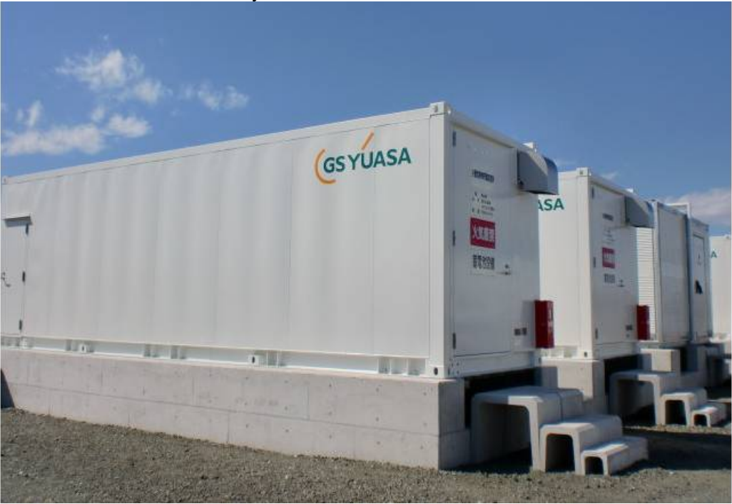
2. Exterior of lithium-ion battery container
