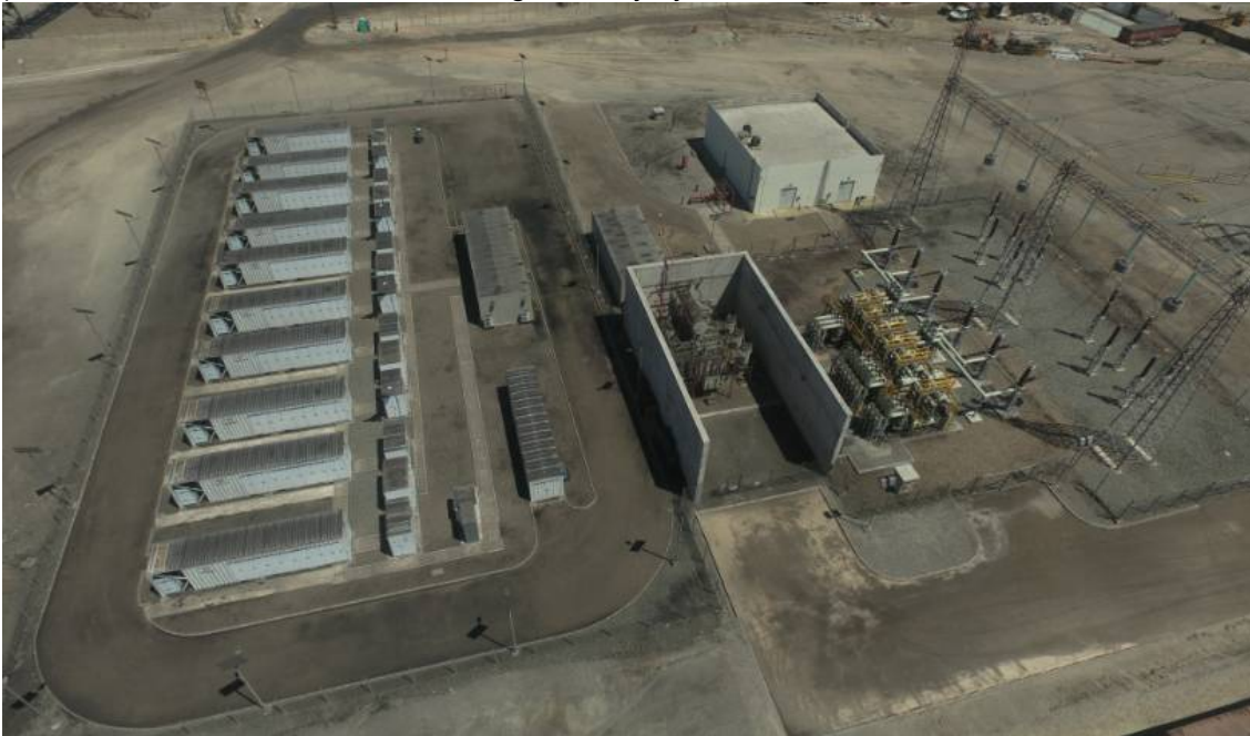
1) The full-view of the lithium-ion storage battery system
