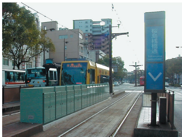
Fig. 1 An installation of overhead line voltage compensator system for streetcars.
