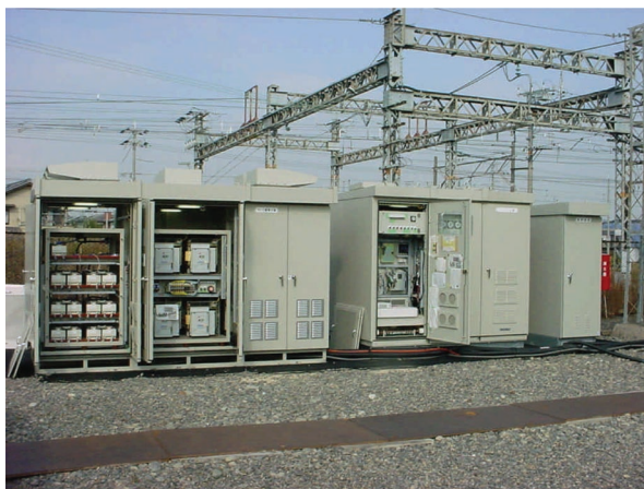
Fig. 33 External appearance of field test for power compensator.
