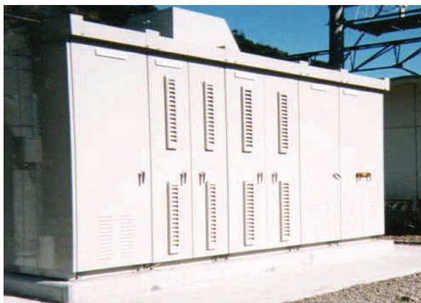
Fig. 4 External appearance of substation support equipment.
