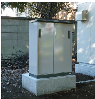
Fig. 4 Battery cabinet installation for charge station for RE-EV.
