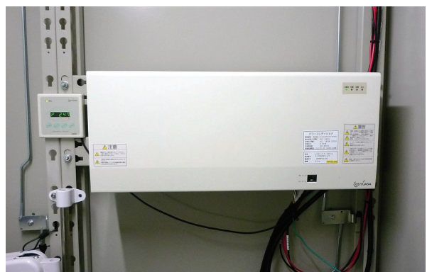
Fig. 3 Power conditioner installation for charge station for RE-EV.
