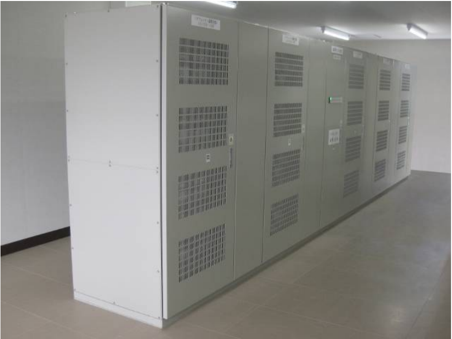
2. Lithium-ion storage battery system installed at Hiraizumi Station
