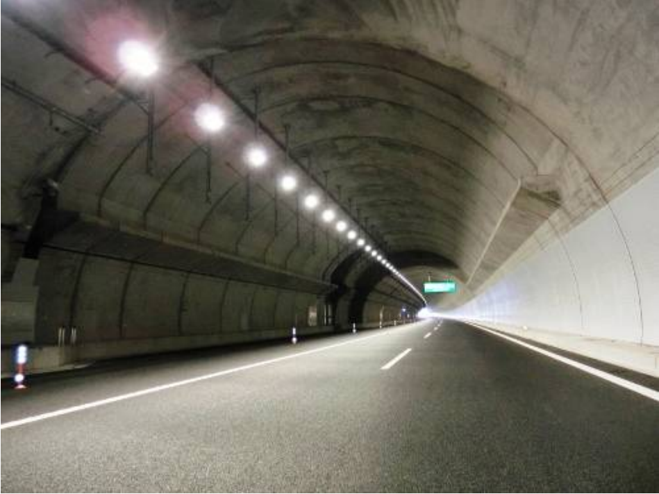
ECO-CERA SR lighting equipment installed in the Fujikawa Tunnel
