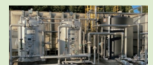
Rainwater treatment facility
