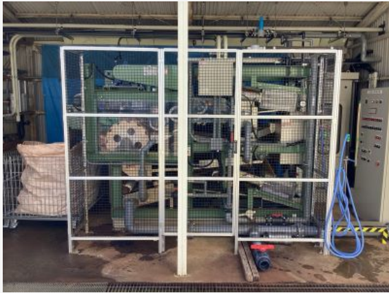
Belt press dewatering machine
